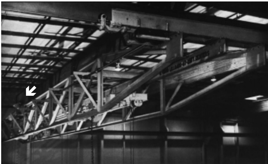
Note the double truss framework with a single bridge girder and tandem drivewheel assembly on the end truck. To place the crane in perspective, note the worker to the rear of the crane. (Photo taken during installation and testing.)
