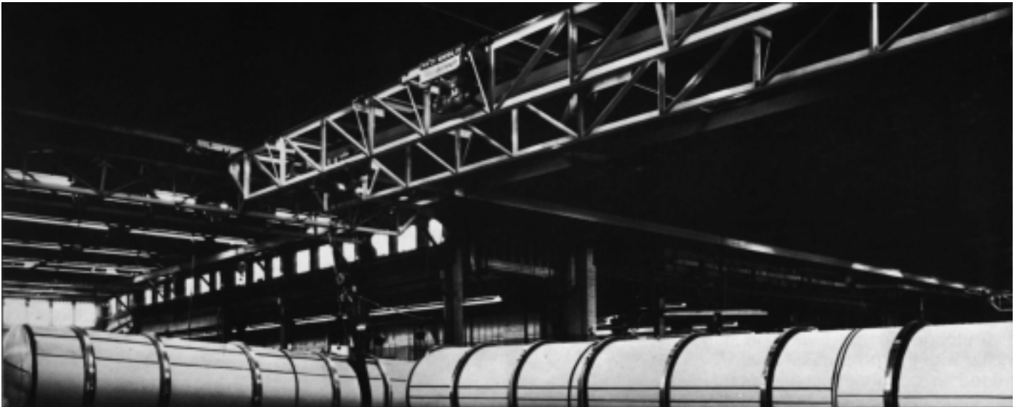
Single girder, double truss crane used in manufacturing plant to handle long, cylindrical tanks. This type of crane fits the long span requirement, yet does not sacrifice headroom or capacity.
